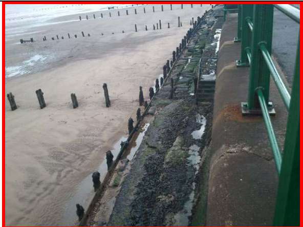
Failed timber groynes and timber breastwork at toe of wall in front of Sandsend (Asset Ref. 1221D901D0702C01)
