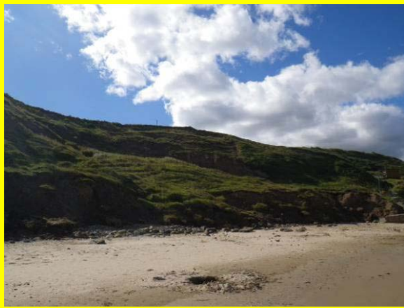
MU24/C A slump of material which is becoming more vegetated and stable (Locally Active)
