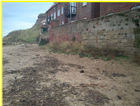
Riparian walls backing sandy beach in east side of harbour, (Asset Ref. 1221D901D0803C09)
