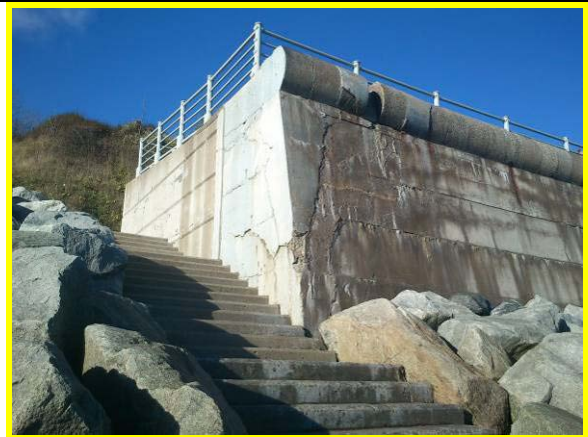
Failing previous repairs at south end of Quarter Deck (Asset Ref. 1221D901D1003C10)
