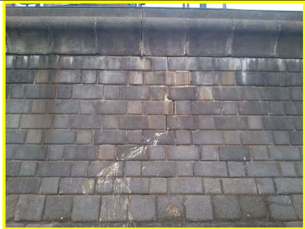
Small vertical crack in wall that has been repaired previously. (Asset ref. 1221D901D1602C06)
