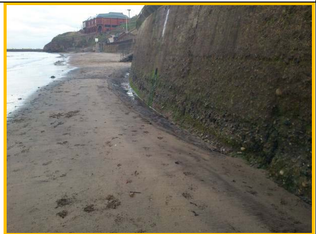
Abrasion damage to wall (Asset ref. 1221D901D0802C14)
