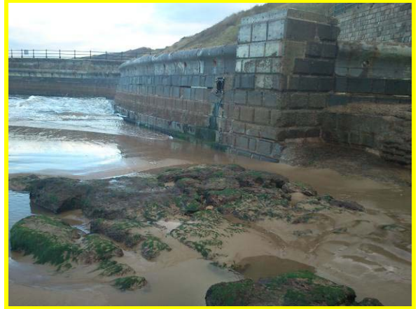
Repaired upper section of upper wall adjacent to re-constructed concrete ramp. (Asset Ref. 1221D901D1303C02)
