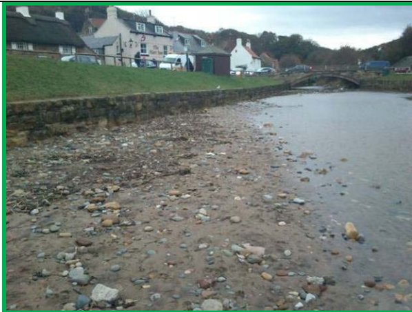
Low masonry wall at east Row Beck, south bank. (Asset Ref. 1221D901D0702C03)
