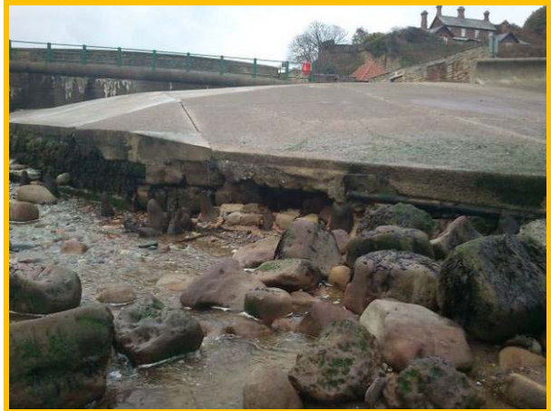
Void under slipway at the north of Sandsend (Asset Ref No.1221D901D0701C02)
