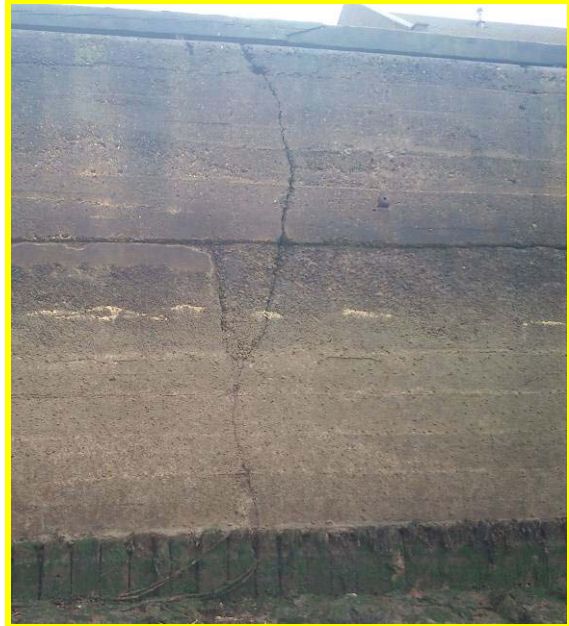
No change to vertical crack extending through the wall photo from 16/10/12, but lower beach exposing timber toe piles. (Asset Ref. 1221D901D1301C19)
