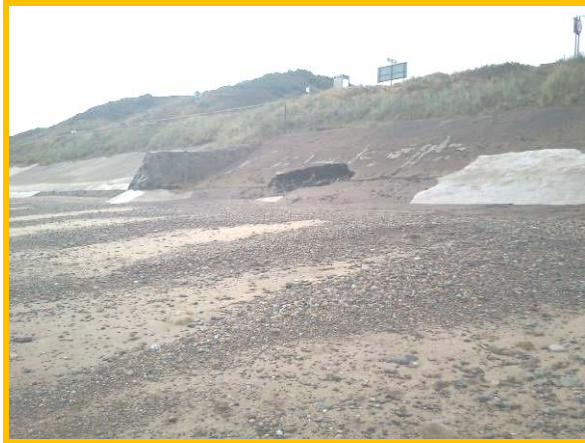
Large void in revetment adjacent to recent patch repair (Asset Ref. 1221D901D0702C02)
