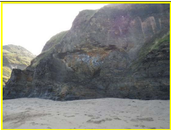
MU7/4 – Toe erosion at the base of the cliff (Locally Active)
