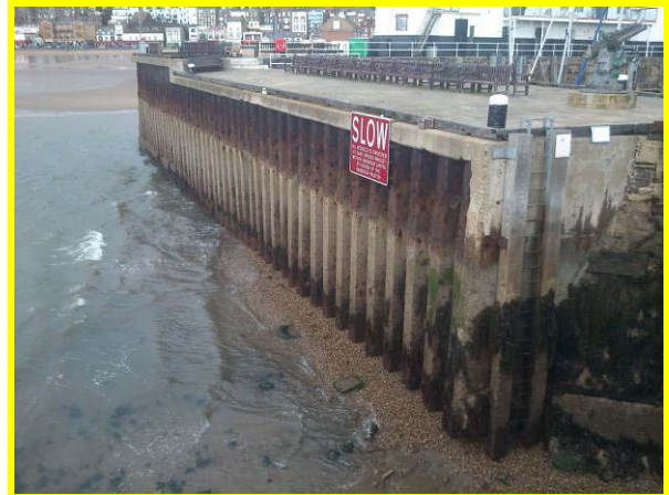
Corroded sheet piles, but overall fair condition (Asset Ref. 1221D901D1301C17)
