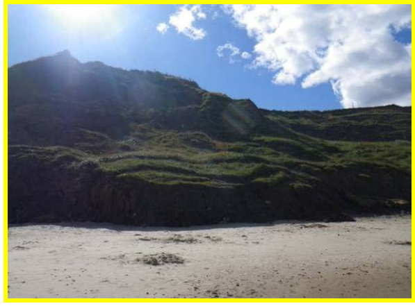
MU24/D Toe slumping which is more stable than during the last inspection (Locally Active)
