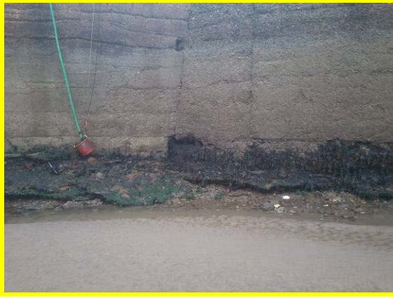
Undermining of toe of concrete encased section at bend where West Pier narrows (Asset Ref. 1221D901D1301C07)
