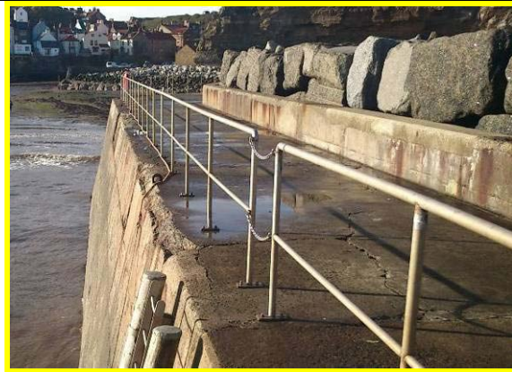
North breakwater promenade and inner face showing cracking in slab and damage to coping. (Asset Ref. 1221D901D0402C01)
