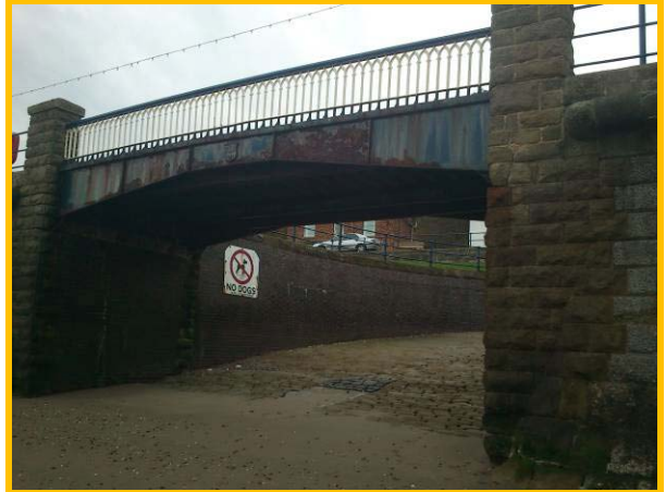
Pedestrian bridge at access slipway from Cargate Hill. Corrosion to bridge and open joints in slipway blocks need attention. (Asset Ref. 1221D901D1602C08)
