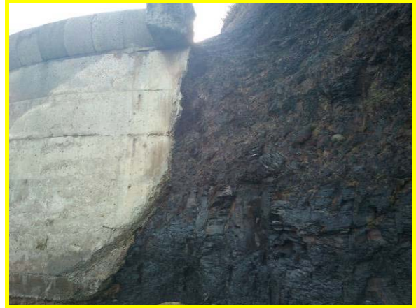
Erosion of cliff adjacent to north end of seawall, 30/10/2012 (Asset Ref. 1221D901D0601C01)
