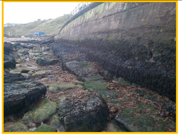
Undermining of toe in section with no rock armour (Asset Ref. 1221D901D0802C03)
