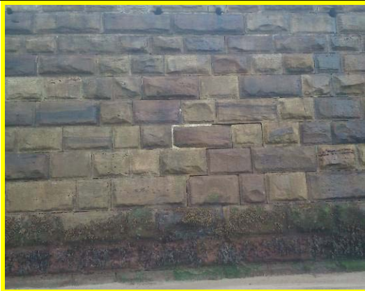
Loose blocks and open joints with failed previous repairs blockwork wall (Asset Ref. 1221D901D1301C27)
