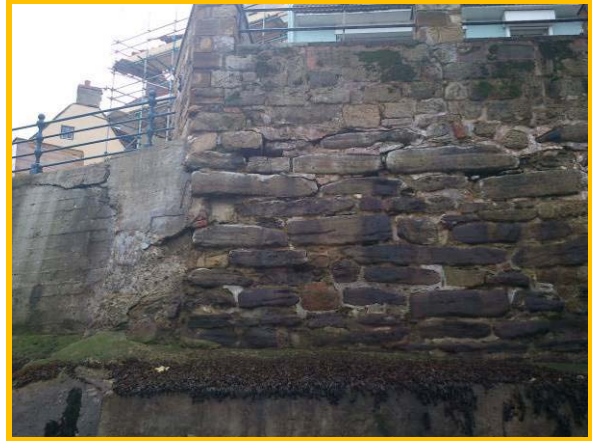
Older sections of harbour wall in need of regular maintenance (Asset Ref. 1221D901D0402C22)
