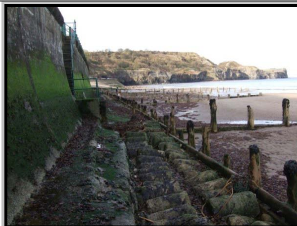
Timber toe of sea wall in a poor state - photo from 2009 (Asset Ref. 1221D901D0702C01)
