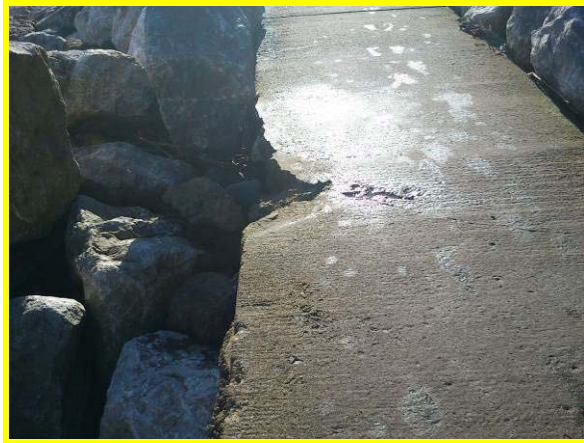
Damage to the walkway / promenade, as also noted in 2009 inspection (Asset Ref. 1221D901D0402C02)
