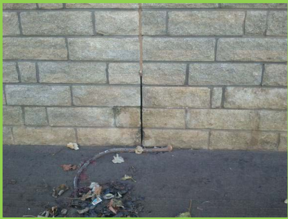
Missing filler in construction joint in new wall north of Peasholm Gap (Asset Ref. 1221D901D1201C06)
