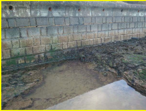
Undermining of wall, with voids at South Bay Pool (Asset Ref. 1221D901D1303C02)
