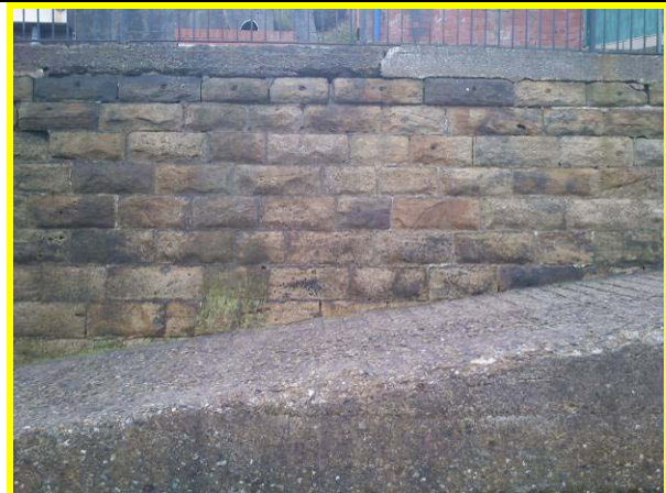
Cracking, mortar loss, damage to capping and localised repairs (Asset Ref. 1221D901D0802C07)
