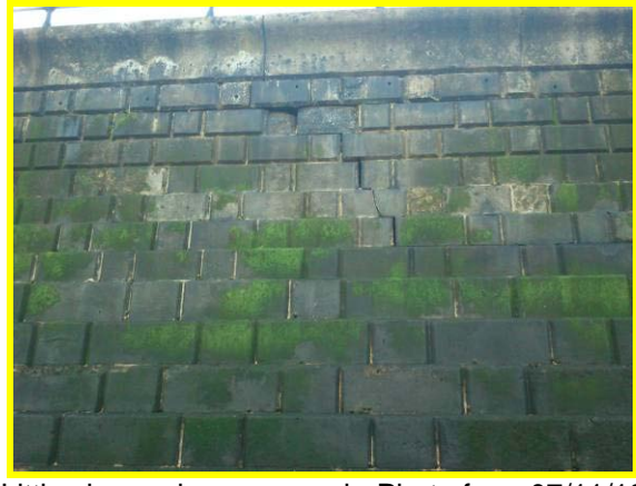
Little change is same crack- Photo from 07/11/12 (Asset Ref. 1221D901D1202C23)
