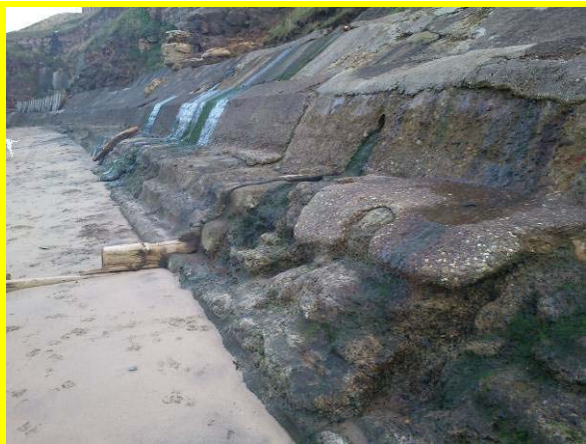
Defence toe suffering abrasion and weathering (Asset Refs. 1221D901D0802C05)
