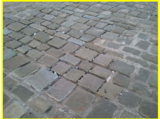
Missing grout in sections of cobbles in slipway (Asset Ref. 1221D901D1602C01)
