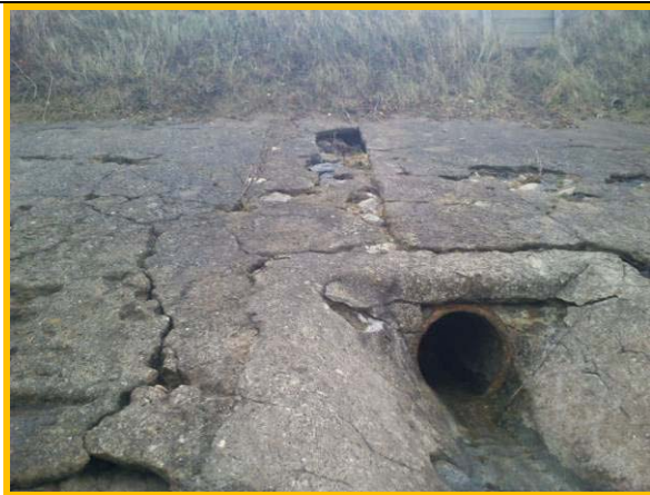
Cracks and voids in surface of concrete revetment (Asset Ref. 1221D901D0702C02)
