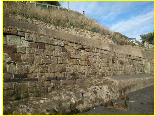
Gaps at joints and missing blocks (Asset Ref. 1221D901D0601C03)
