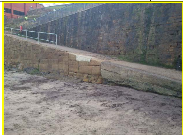
Cracking, mortar loss and damaged blocks (Asset Ref. 1221D901D0802C06)
