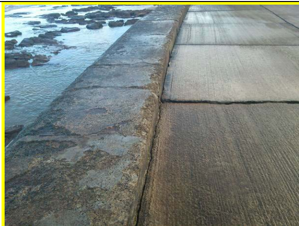
Missing joint sealant in gaps promenade slabs (Asset Ref. 1221D901D1303C02)
