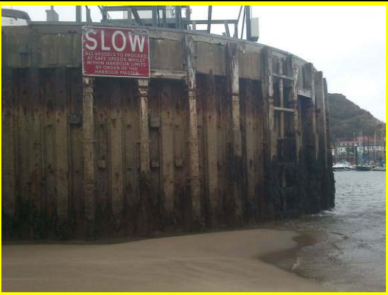
Corroded sheet piling and damaged timber fenders at end of West Pier (Asset Ref. 1221D901D1301C18)
