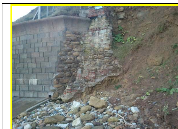
Tie in of Pumping station defences at north end (Asset Ref. 1221D901D1402C02)
