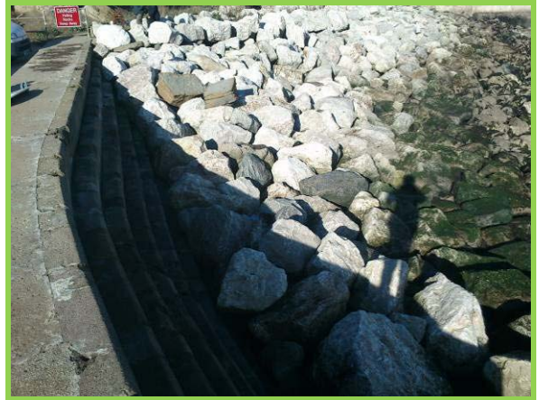
Rock armour which is in good condition adjacent to stepped wall at end of Cowbar Lane. (Asset Ref. 1221D901D0402C02)
