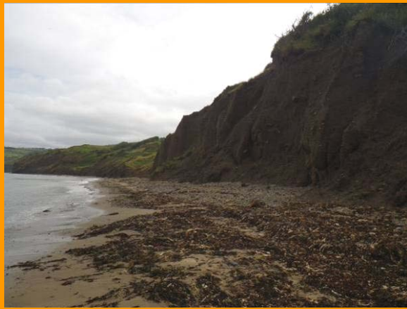
MU175 has been subject to marine erosion at the toe of the cliff (Partly Active)
