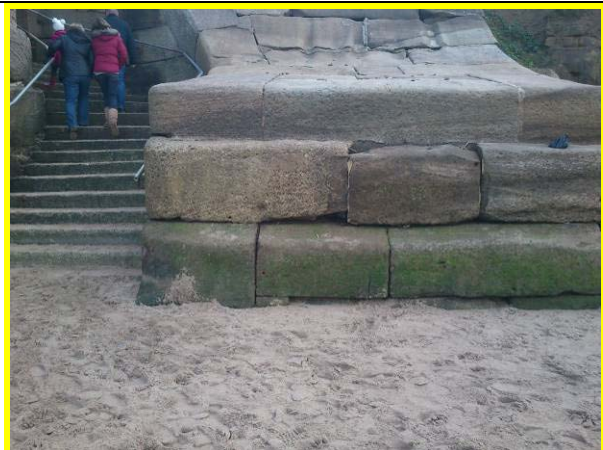
Evidence of recent movement of central block (Asset Ref. 1221D901D0802C12)
