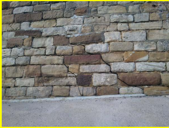
Diagonal cracks in wall (Asset Ref. 1221D901D0601C03)
