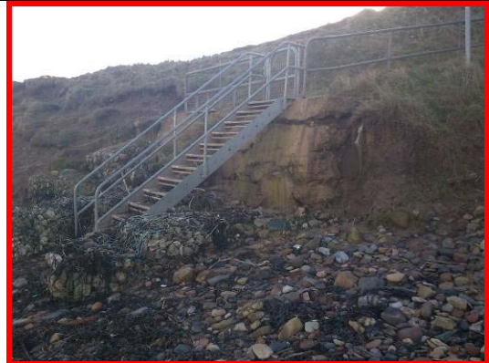
(Failed gabion baskets at south beach access)
