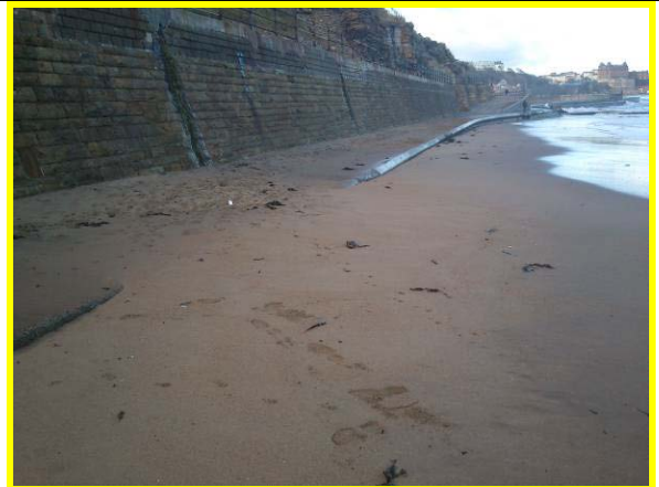
High beach covering lower wall at Holbeck Gardens (Asset Ref. 1221D901D1304C02)
