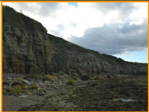
MU23/A Erosion of the toe (Partly Active)
