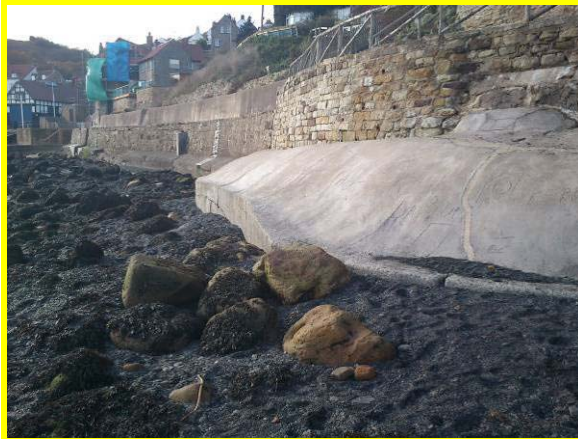
Repaired vertical cracks to toe of wall, and horizontal cracks holding (Asset Ref. 1221D901D0601C06)
