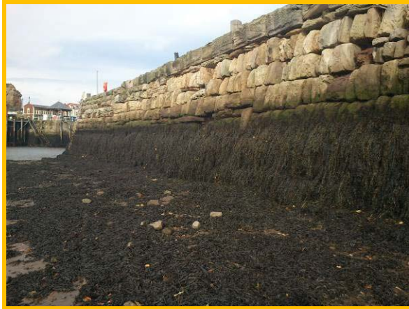
Heavily weather blocks on south side of Tate Hill pier (Asset Ref. 1221D901D0803C08)
