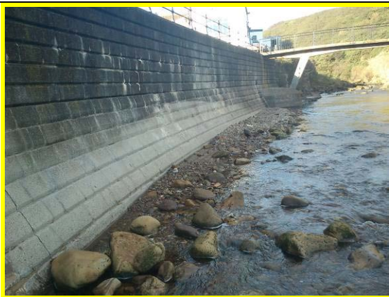
Wall on south side of Scalby Beck in fair condition (Asset Ref. 1221D901D1201C01)
