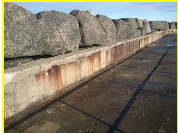
North breakwater outer crest wall showing horizontal cracking and rust staining. (Asset Ref. 1221D901D0402C01)
