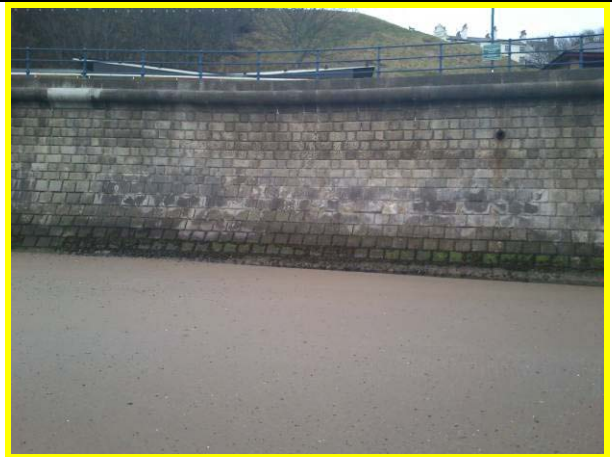
General view of wall showing area of damaged blocks and previous repairs to coping / splash beam. (Asset ref. 1221D901D1602C07)
