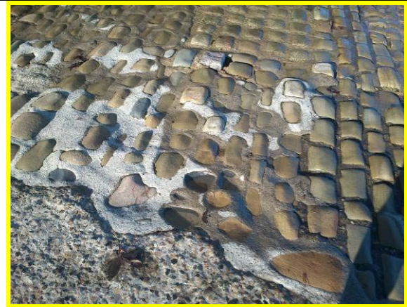
Missing cobbles and mortar in slipway, with evidence of previous repair work with contrasting colour mortar. (Asset Ref. 1221D901D1003C05)
