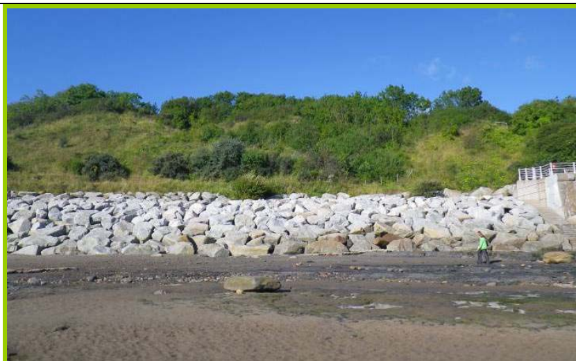
MU17/1 The defended toe and heavily vegetated slopes show that the unit has been stable (Inactive)
