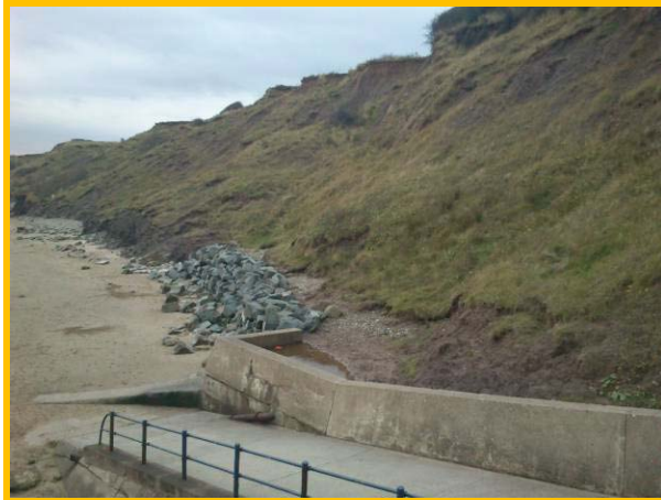
General view of rock armour at interface with natural cliff (Asset Ref. 1221D901D1602C02)
