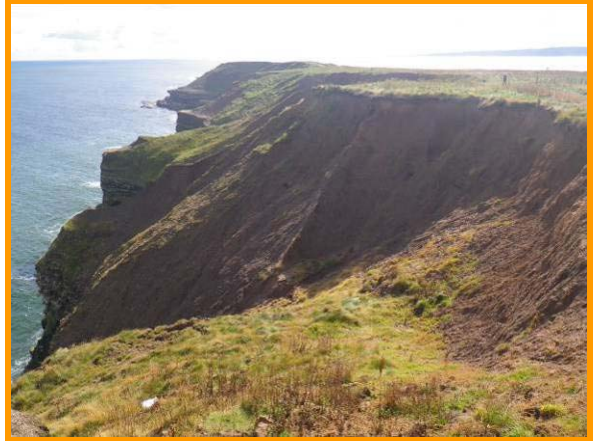
MU27/BA The failure which had been observed in 2009 is now beginning to stabilise (Partly Active).
