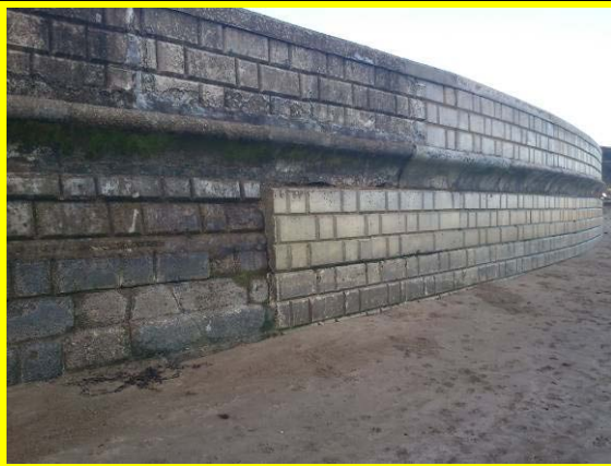
Recent repairs to areas of front face of wall. Asset Ref. 1221D901D1201C04
