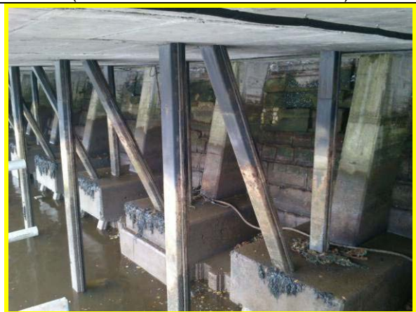
View of original quay wall and deck support piles near north end of Asset Ref. 1221D901D0803C06
