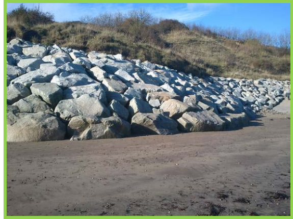
Tightly packed rock armour (Asset Ref. 1221D901D1003C07)
