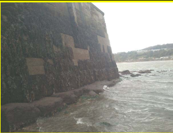
Erosion at toe, south end of East Pier. (Asset Ref. 1221D901D1301C16)
