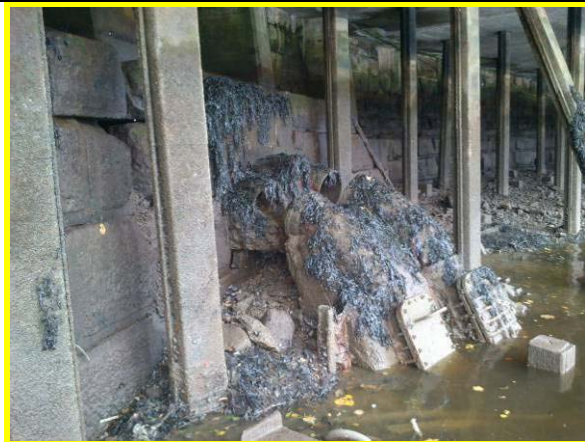
Broken outfall between promenade supports under pier (Asset Ref. 1221D901D0803C06)
