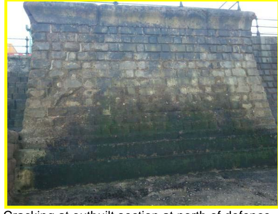
Cracking at outbuilt section at north of defence – photo from 07/11/2012. (Asset Ref. 1221D901D1201C08)
