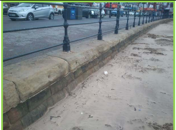
High beach level along sea wall running in front of Foreshore Road, South Bay (Asset Ref. 1221D901D1301C15)
