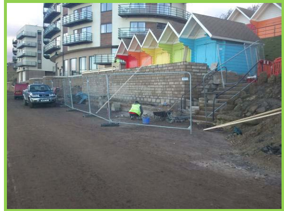
New rear property boundary wall under construction at south end of Asset Ref. 1221D901D1201C05
