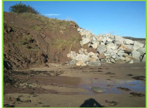
Erosion adjacent to south end of rock armour. November 2012 (Asset Ref. 1221D901D1003C07)
