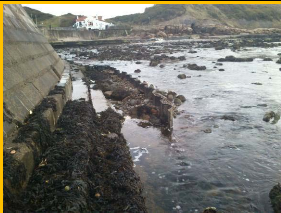
Exposed toe at Sea Life Centre. Note missing infill apron behind end of sheet pile toe. (Asset Ref. 1221D901D1201C02)
