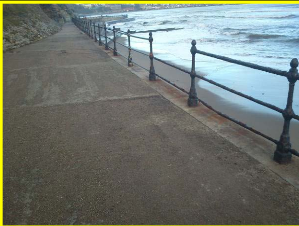
Corroded handrail with missing section on upper level prom (Asset Ref. 1221D901D1304C02)
