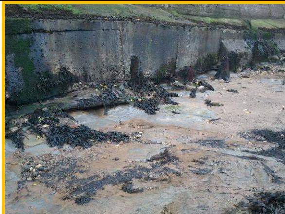
Undercutting at the toe of some parts of the harbour wall (no change since 2009) (Asset Ref. 11221D901D0402C22)
