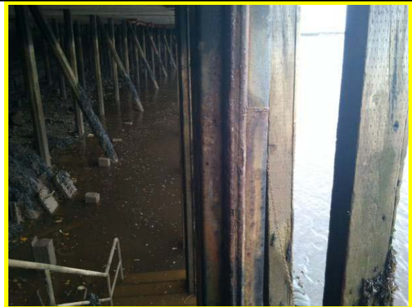
Corrosion to deck support columns (Asset Ref. 1221D901D0803C06)
