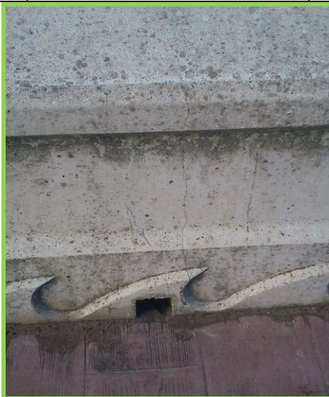
Example of crack through centre of wave wall – (Asset Ref. 1221D901D1202C03)
