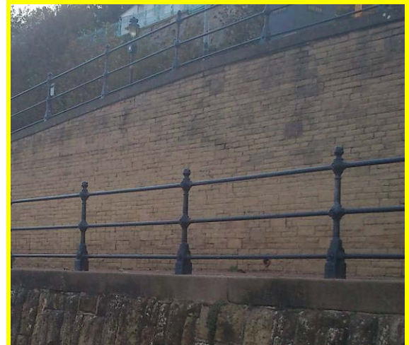
Second stage wall, with crack, 16/10/12 (Asset Ref. 1221D901D1301C09)
