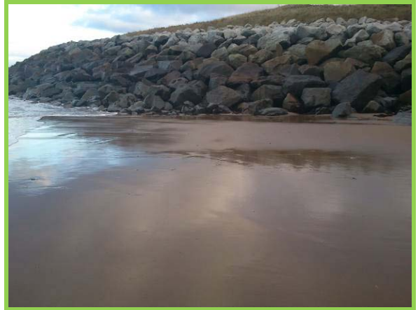
Rock armour revetment at Holbeck landslide (Asset Ref. 1221D901D1304C01)
