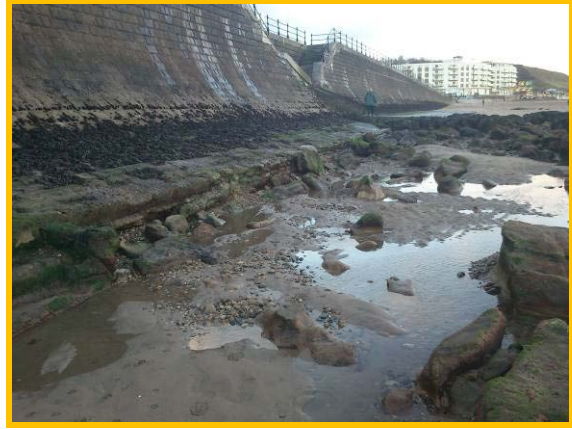
Low beach levels exposing toe apron (Asset Ref. 1221D901D1201C21)
