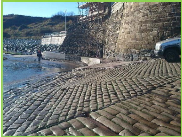
Central Slipway in overall good condition (Asset Ref. 1221D901D1003C05). (Masonry wall forming property foundations to rear in fair condition -1221D901D1003C06).
