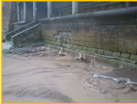
Loss of stone facing and undermining of the toe on lower level wall (Asset Ref. 1221D901D1302C01)
