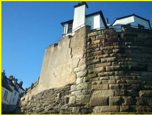
Loose render on property wall to north side of slipway (Asset Ref. 1221D901D1003C04)
