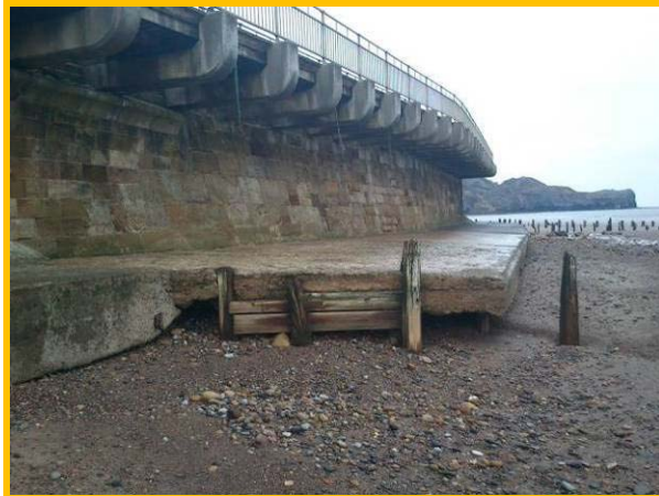
Masonry blockwork sea wall with cantilevered footway, showing large void under toe apron and failed groynes. (Asset Ref. 1221D901D0702C04)
