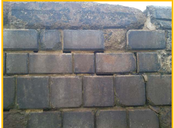
Cracks in wall and loose blocks adjacent to slipway 08/11/12. (Asset Ref. 1221D901D1602C01)
