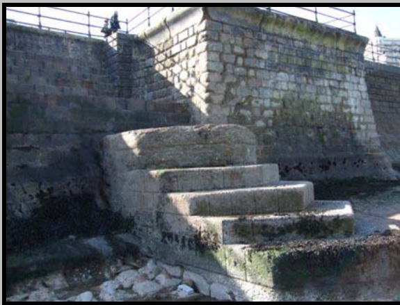
Cracking outbuilt section at north of defence – photo from 2009. (Asset Ref. 1221D901D1201C08)
