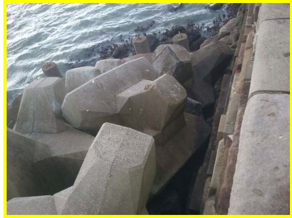
South end of harbour arm showing potential lack of armour fill Photo taken 16/10/2012 (Asset Ref. 1221D901D1301C01)
