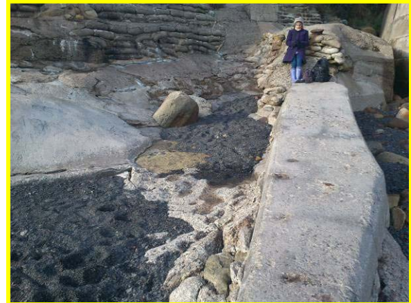
View of northern end of wall with cracked concrete bagwork. (Asset Ref. 1221D901D0601C06)
