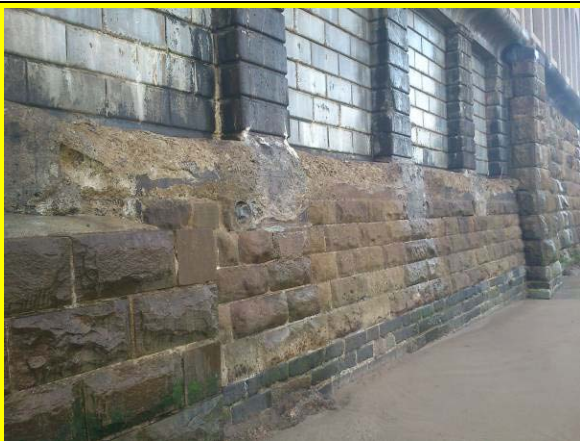
Abraded and spalling concrete capping to original wall below infilled openings (Asset Ref. 1221D901D1301C29)
