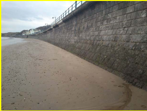
General view of wall showing repaired coping wave return blocks and abrasion damage to blocks near beach level. (Asset Ref. 1221D901D1602C08)
