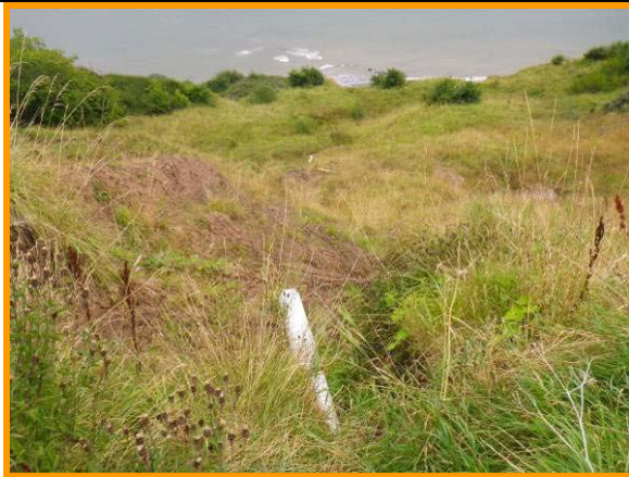
MU17/2 The land drains from the adjacent fields are draining on to the cliff and causing instability (Partly Active).
