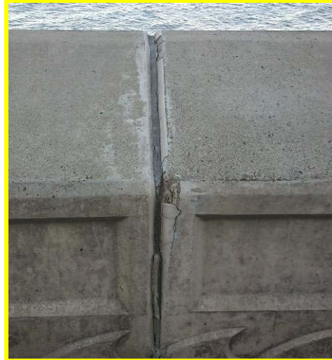
Expansion joint in crest wall needs repair (Asset Ref. 1221D901D1202C02)
