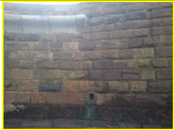
Repaired splash beam, but cracks in blockwork below (Asset Ref. 1221D901D1301C28)
