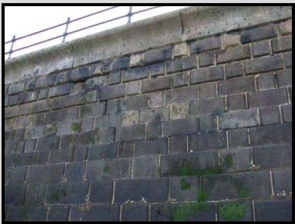
Example of cracking Photo from 2009 (Asset Ref. 1221D901D1202C23)
