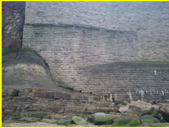
Cliff protected with block/brickwork undercutting at interface with cliff requires repair (Asset Refs. 1221D901D0802C09)
