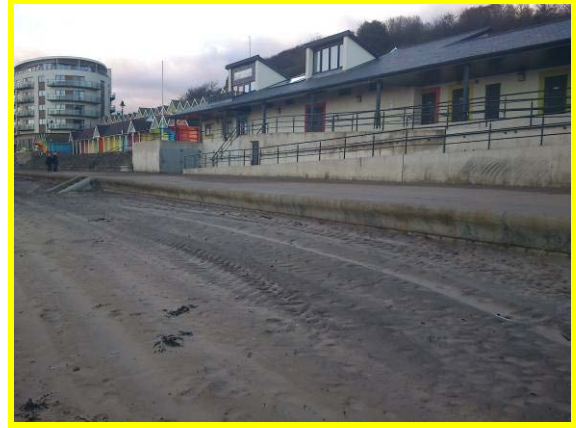
High beach in front of new rear wall at beach management centre, (Asset Ref. 1221D901D1201C15)
