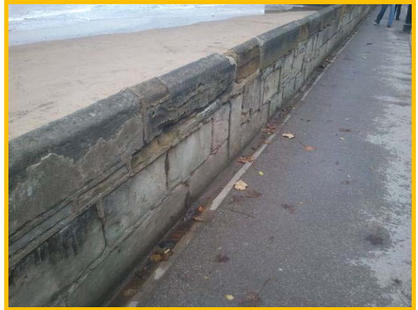
Erosion and weathering to limestone blocks in crest wall (Asset Ref. 1221D901D1301C26)
