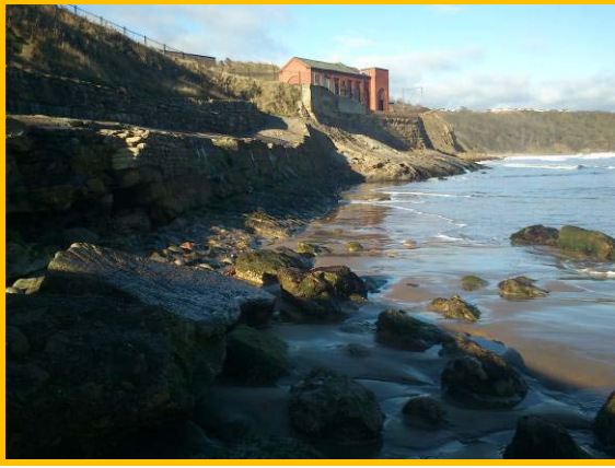
Large voids to makeshift defences to the south of the pumping station (Asset Ref. 1221D901D1402C04)
