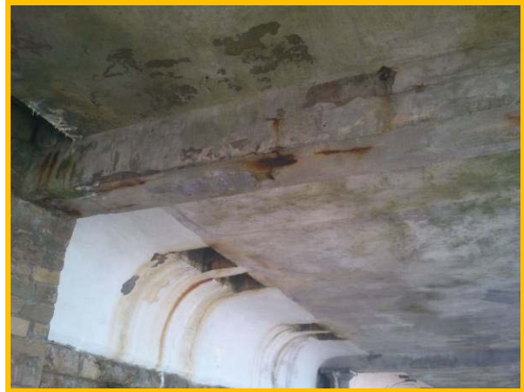
Cracking and corrosion to beams supporting upper level prom. (Asset Ref. 1221D901D1302C01)
