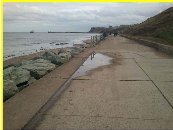
Promenade looking south east showing cracks in slabs and standing water (Asset Ref. 1221D901D0801C01)
