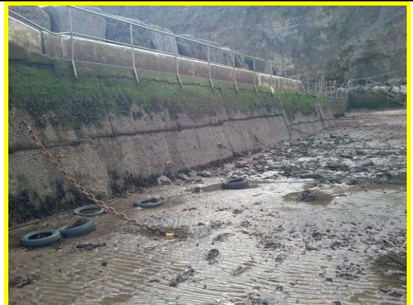
Exposure of aggregate and construction joints in south breakwater inner face. (Asset Ref. 1221D901D0403C03)
