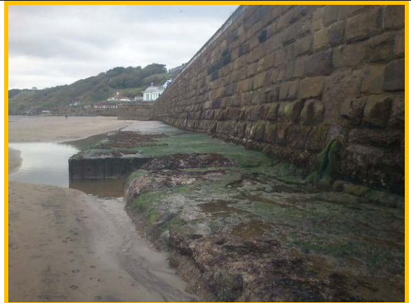
Exposed and abraded toe apron at the Spa (Asset Ref. 1221D901D1301C27)
