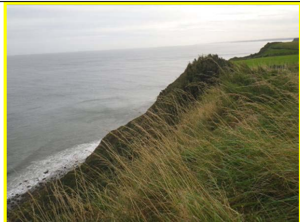
MU18/4 Vegetated overall but with localised erosion (Locally Active)
