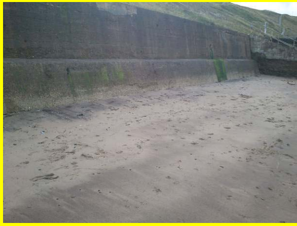
Patchwork repairs to capping holding (Asset Ref. 1221D901D0802C04)
