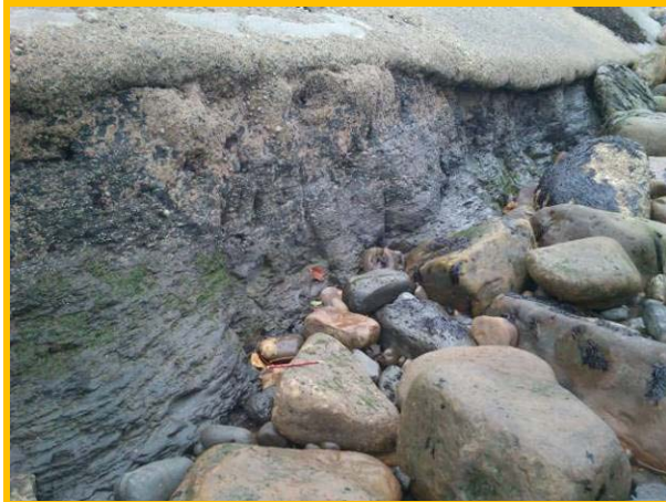
Displaced toe armour, undercutting to concrete revetment and abrasion damage to revetment (Asset Ref No.1221D901D0701C02)
