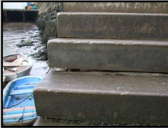
Washout behind steps – photo from 2009 (Asset Ref. 1221D901D1301C16)
