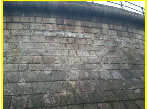
Horizontal crack in upper wall on southern promontory. (Asset Ref. 1221D901D1602C05)
