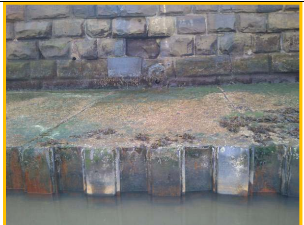
Loose blocks set back in void at toe of wall (Asset Ref. 1221D901D1301C27)
