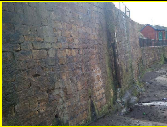
Cracking, mortar loss and vegetation growth due to leaking pipe (Asset Ref. 1221D901D0802C06)
