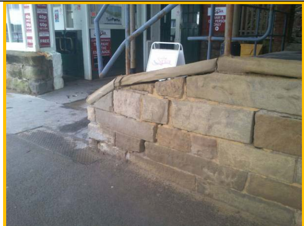
Weathering and loss of joints in stone wall at back of high level prom by cliff railway (Asset Ref. 1221D901D1302C01)
