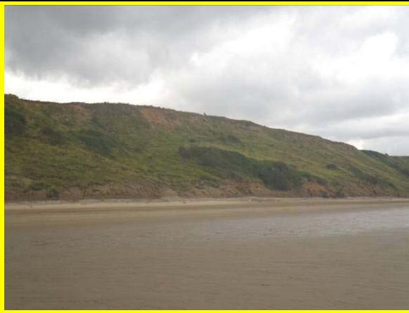
MU29/AE The slope is well vegetated with erosion at the toe and headscarp (Locally Active)
