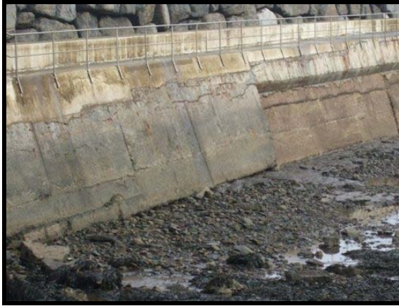
Undercutting to landward facing of north breakwater (photo from 2009 inspection) (Asset Ref. 1221D901D0402C01)
