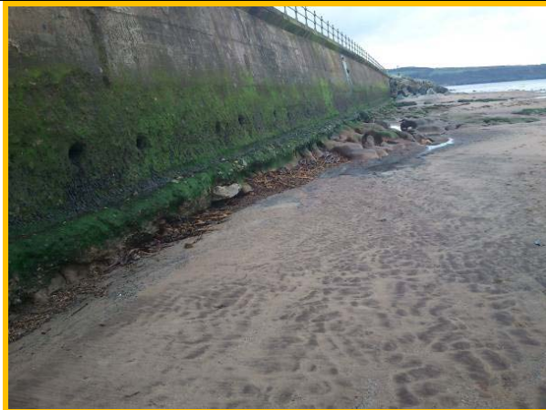
Undermining of toe in section with no rock armour (Asset Ref. 1221D901D0802C01)
