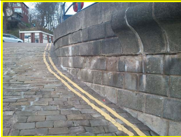
Damaged blocks at ramp with evidence of previous repairs. (Asset ref. 1221D901D1602C06)
