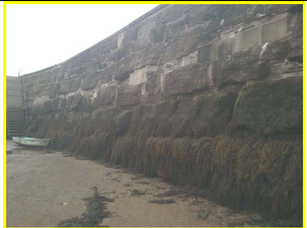
Open joints between blocks in inner face of east Pier below repaired section. (Asset Ref. 1221D901D1301C16)
