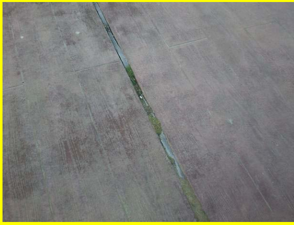
Joints in promenade slab needing re-sealing (Asset Ref. 1221D901D1202C02)
