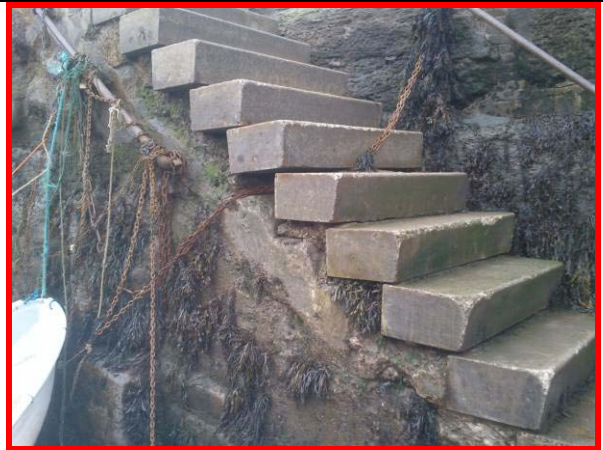
Washout behind steps – 16/10/2012 (Asset Ref. 1221D901D1301C16)
