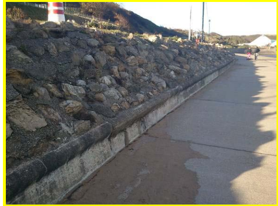
Grouted revetment behind prom has missing infill and voids in several locations Asset Refs. 1221D901D1201C25 & C04
