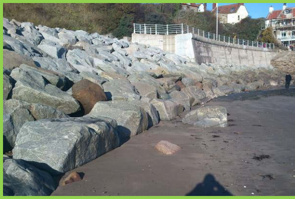
Apparently displaced rock armour units (Asset Ref. 1221D901D1003C07)
