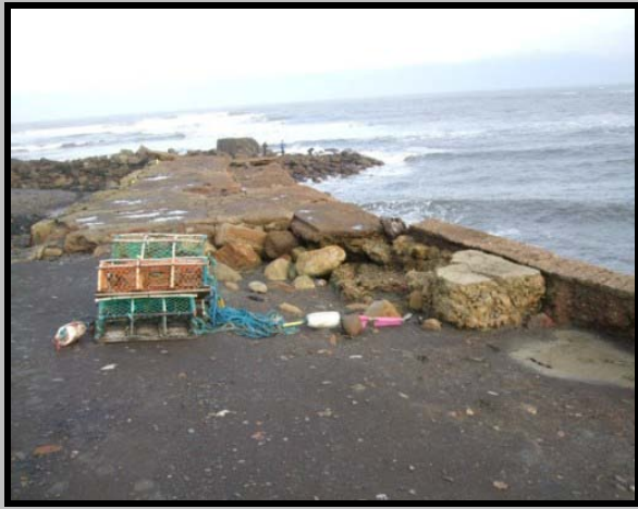
Looking at the end of the breakwater with evidence of erosion and failure in 2009 (Asset Ref. 1221D901D0502C01)
