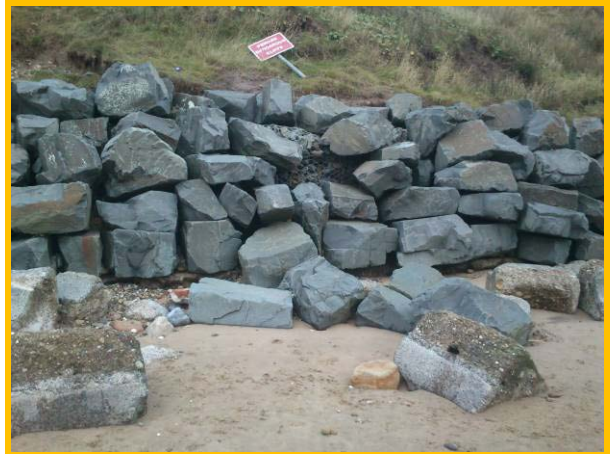
Collapsed section of rock and slumping cliff behind. (Asset Ref. 1221D901D1602C02)
