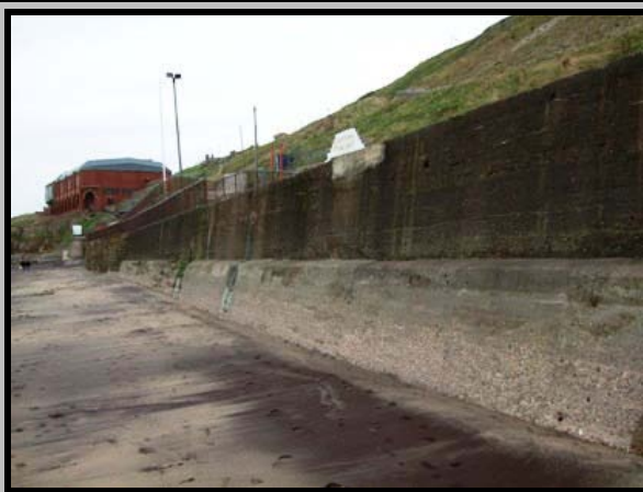
Overview of asset, looking south. Patchwork repairs to capping visible – photo from 2009. (Asset Ref. 1221D901D0802C04)
