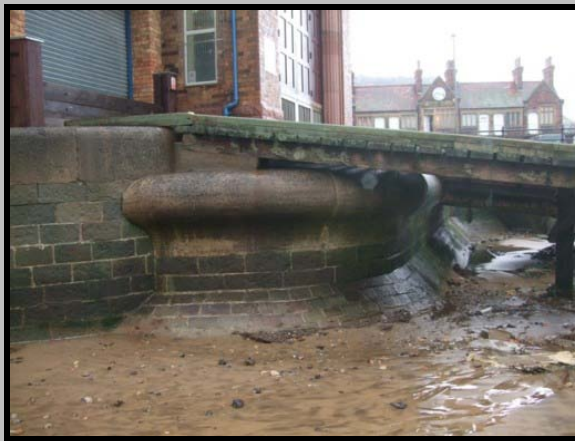
View of blockwork wall beneath life boat station Photo from 2009 (Asset Ref. 1221D901D1301C08)
