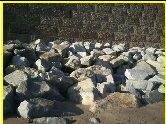
Section of rock armour with gaps / displaced units in front of 2001 seawall. (Asset Ref. 1221D901D1003C01)
