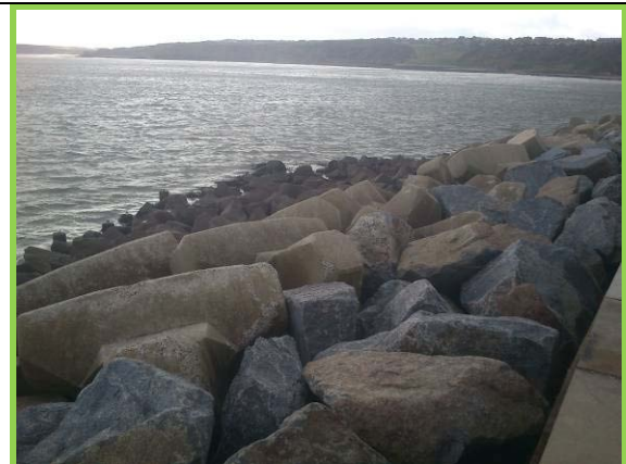
Tightly packed rock armour, Accropodes rock toe blanket and concrete toe piles seaward of East Pier harbour wall (Asset Ref. 1221D901D1301C01)
