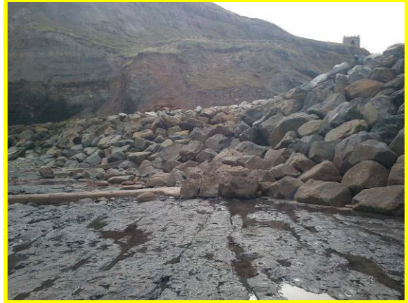
Rock armour at interface between east pier and Abbey cliff (Asset Ref. 1221D901D0803C05)
