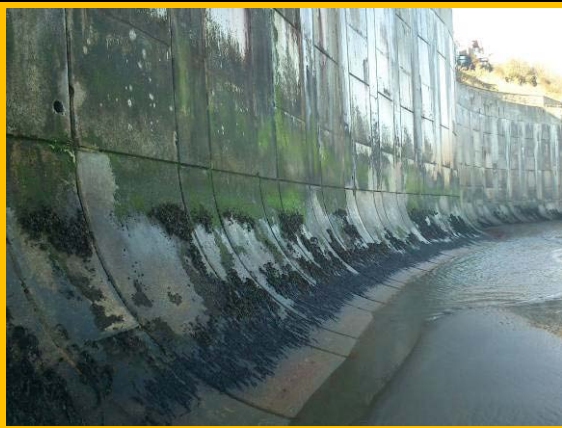
Large vertical wall at Robin Hood's Bay in poor condition (Asset Ref. 1221D901D1003C02)
