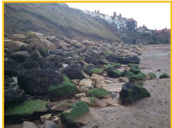
Displaced rock armour and damaged revetment at the Haggerlythe inside harbour adjacent to east pier (Asset Ref. 1221D901D0803C05)
