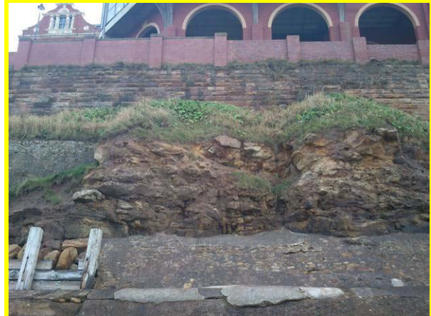
Mortar loss and vegetation growth on upper wall (Asset Ref. 1221D901D0802C15)
