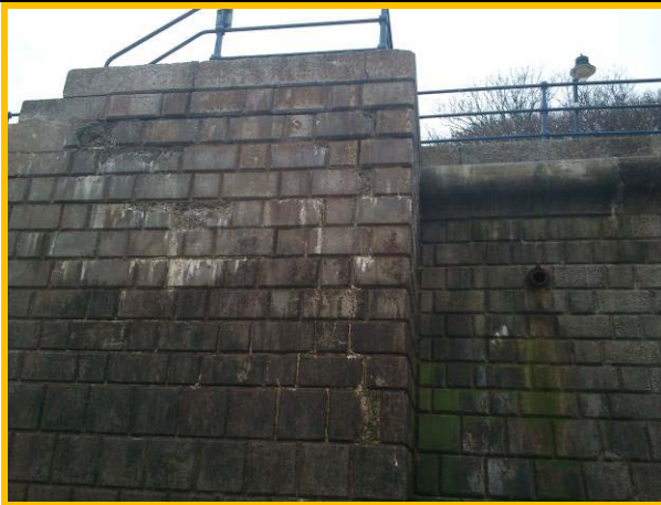
Sea wall with minor, localised defects (Asset Ref. 1221D901D1602C07)
