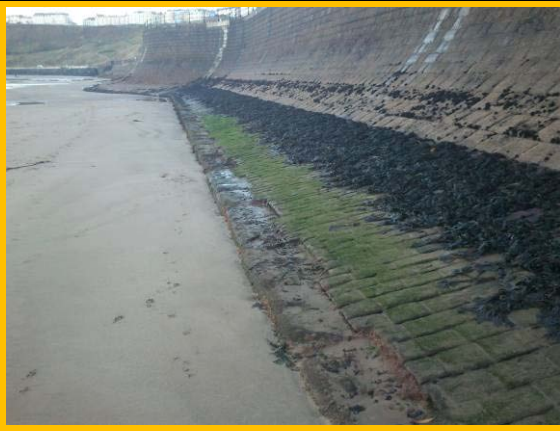
Exposed toe – with missing blocks (Asset Ref. 1221D901D1201C21)
