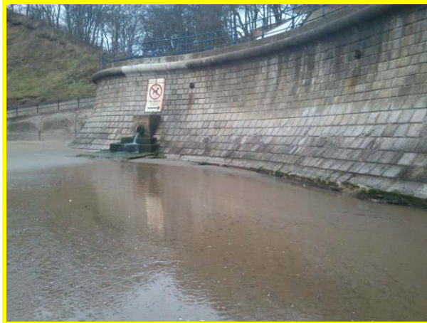
View of south end of wall and discharge from outfall. Damaged toe blocks to wall on right. (Asset Ref. 1221D901D1602C05)
