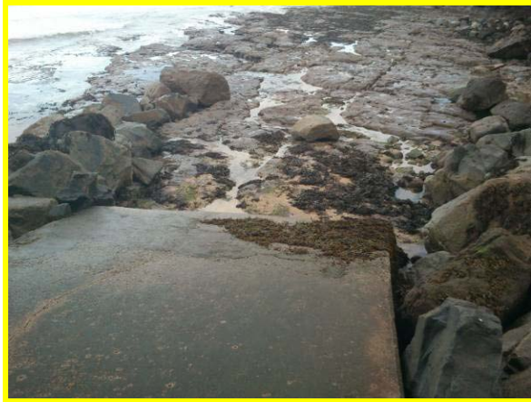
Vertical drop off ramp at south end of Holbeck revetment (Asset Ref. 1221D901D1304C01)
