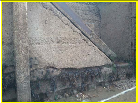
Cracks to concrete facing and exposed toe to steps on West Pier (Asset Ref. 1221D901D1301C18)
