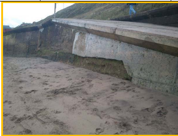
Loss of wall facing and damage to encasement repair (Asset ref. 1221D901D0802C14)
