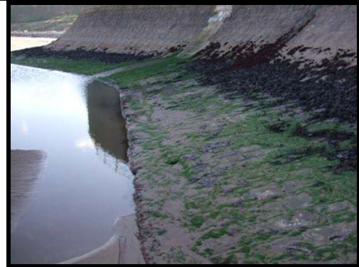
Exposed toe – photo from 2009 (Asset Ref. 1221D901D1201C21)
