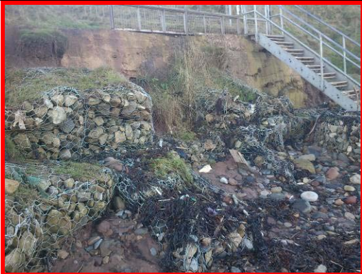
(Failed gabion baskets at south beach access)
