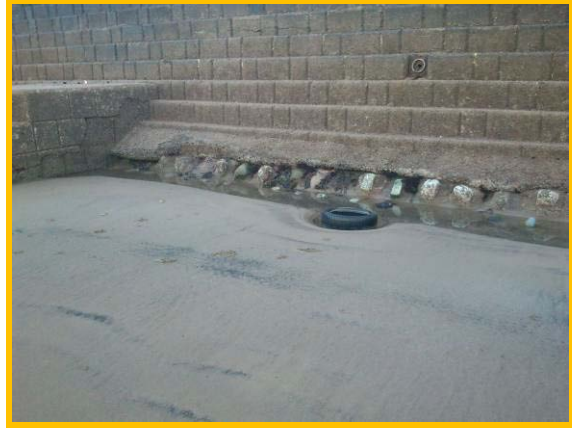
Looking north, showing eroded undermined toe (Asset Ref. 1221D901D1201C08)
