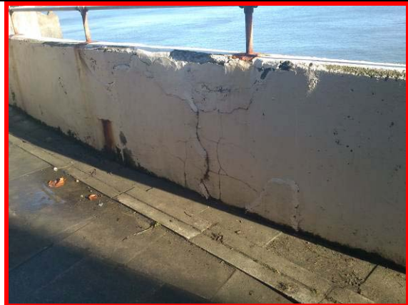
Crest wall in locally very poor condition (Asset Ref. 1221D901D1003C02)
