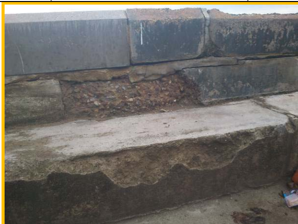
Loose blocks and cracking in crest wall previous repairs (Asset Ref. 1221D901D1301C27)
