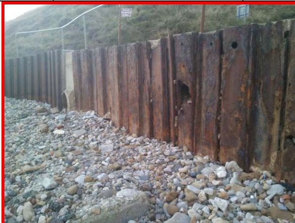
Centre section of sheet piling below Sailing Club house in failed condition. (Asset Ref. 1221D901D1601C03)
