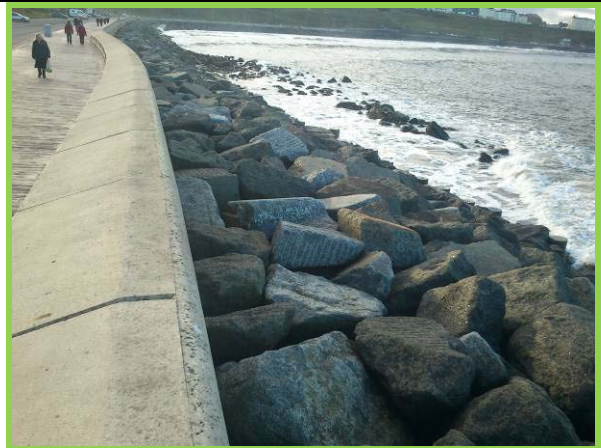
Overview of rock armour with concrete piles at toe visible (Asset Refs. 1221D901D1202C04)
