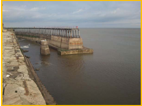
South end of outer east breakwater extension arm, where failed toe piling has been replaced with precast concrete panels. (Asset Ref. 1221D901D0803C04)
