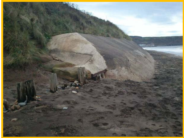
Repair at east end of the concrete revetment since 2009 inspection (Asset Ref. 1221D901D0702C02)
