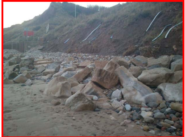
Debris from failed defence and former slope stabilisation at Sailing Club. (Asset Ref. 1221D901D1601C02)
