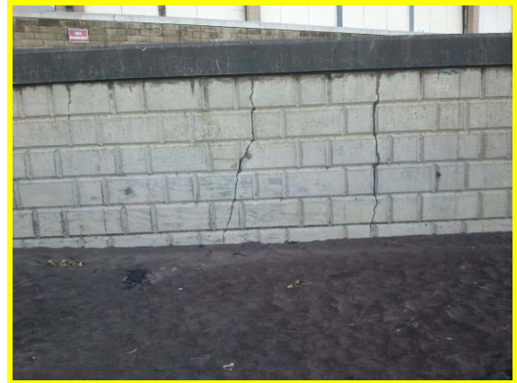
Full height cracks in wall north of Peasholm Gap ramp (Asset Ref. 1221D901D1201C06)
