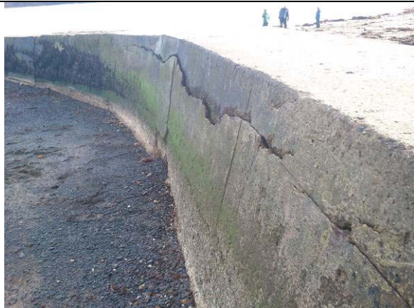
Large horizontal crack to breakwater (Asset Ref. 1221D901D0601C02)
