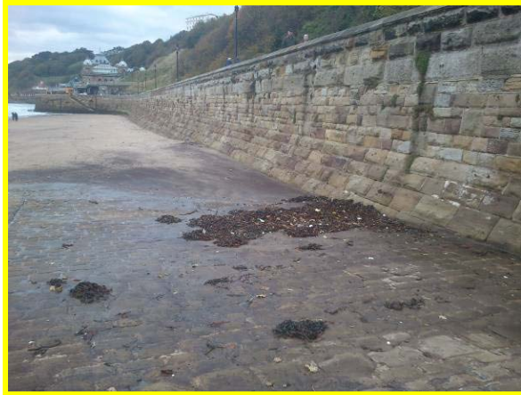
General view of defence at Spa Chalet (Asset Ref. 1221D901D1301C26)
