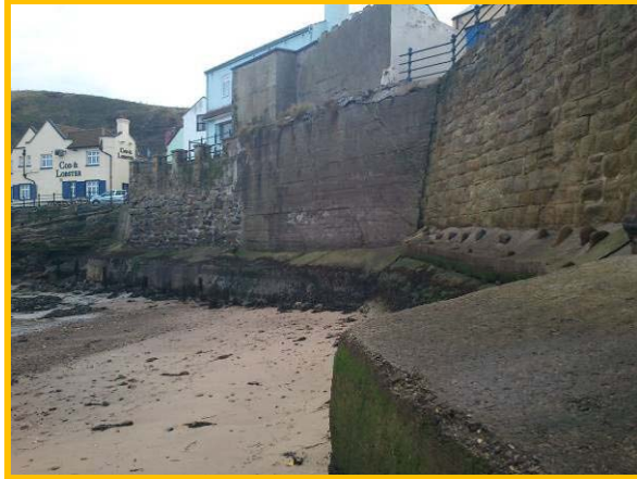
Cracks throughout wall and undercutting of toe (Asset Ref. 1221D901D0402C22)
