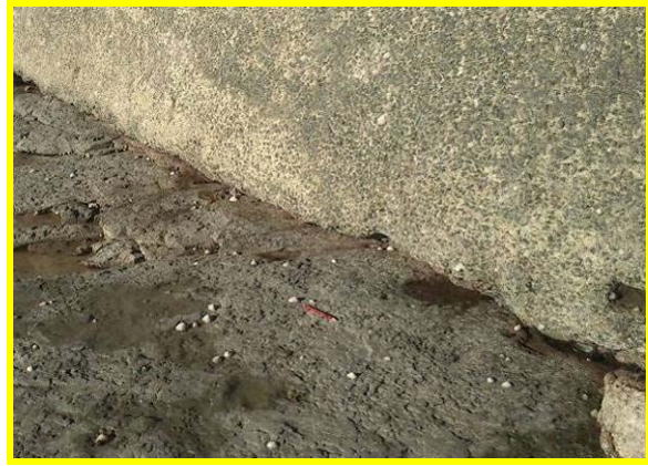
Undercutting at landward facing of north breakwater (30/12/2012) (Asset Ref. 1221D901D0402C01)
