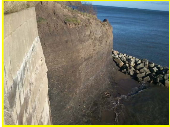
Short section of undefended cliff (Asset Ref. 1221D901D1003C03)
