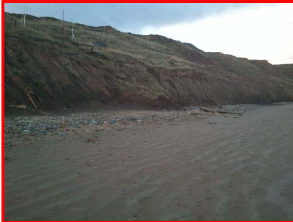
Debris from former slope stabilisation works being eroded at Filey sailing club boat park (Asset Ref. 1221D901D1601C01)
