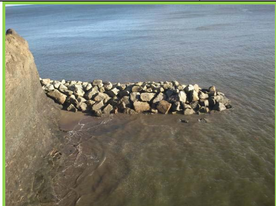
Rock armour extension at the interface between defended and undefended section. (Asset Ref. 1221D901D1003C01)
