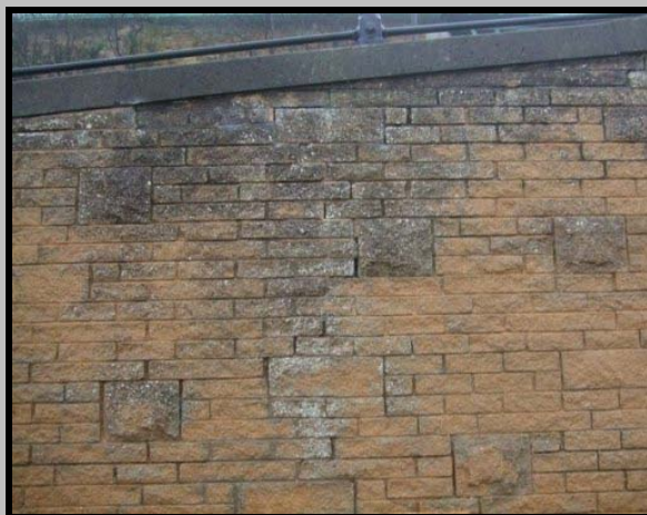
Vertical crack to second wall protecting road. Photo from 2009 (Asset Ref. 1221D901D1301C09)
