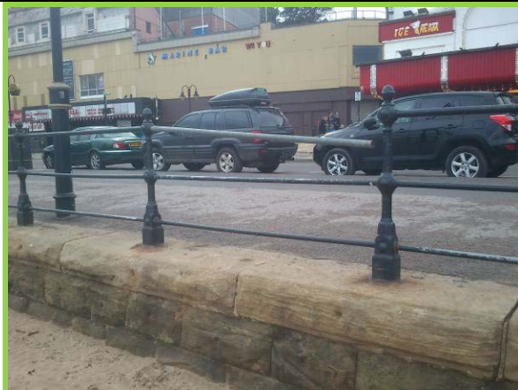
Damaged handrail above wall (Asset Ref. 1221D901D1301C22)
