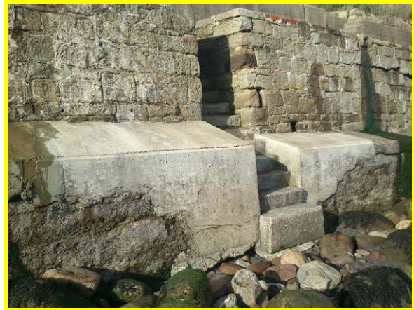
Undercutting of toe adjacent to steps (Asset Ref. 1221D901D0601C03)
