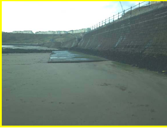
Low beach levels exposing toe apron (Asset Ref. 1221D901D1201C07)
