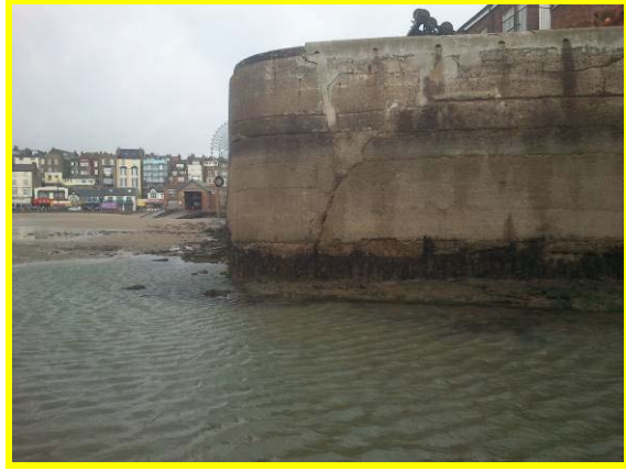
Cracks and repairs in concrete encasement section at narrowing of West Pier (Asset Ref. 1221D901D1301C07)
