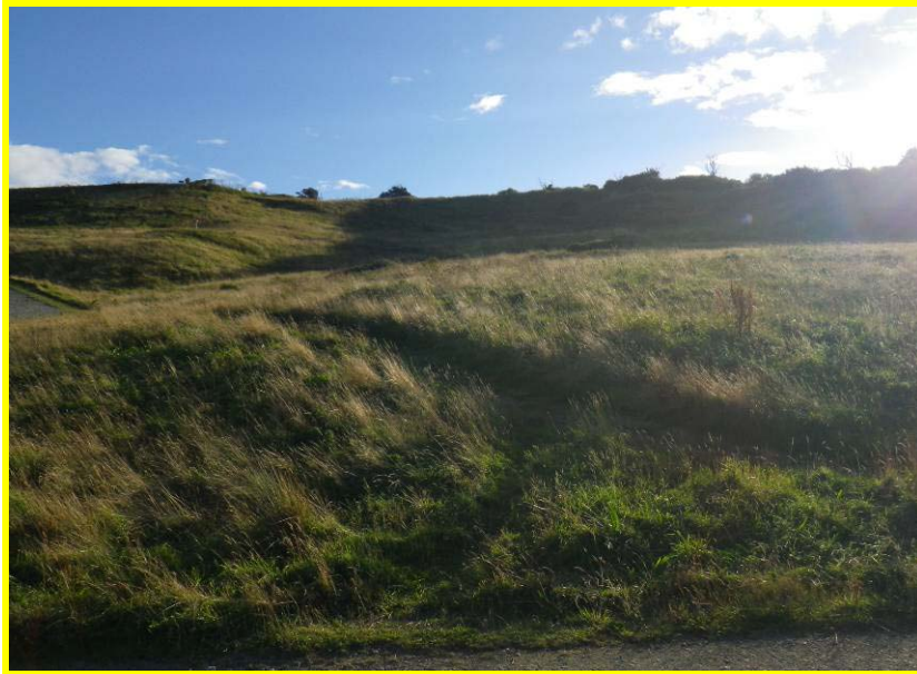
MU22/8 Localised activity at the headscarp of the Holbeck Hall landslide run-out (Locally Active)
