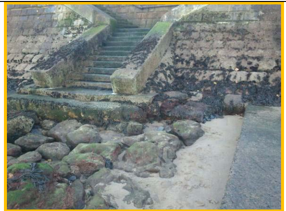
Erosion and undermining at steps at south end of Asset Ref. 1221D901D1201C07
