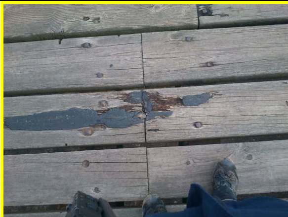
Evidence of rot in ends of timber desk on West Pier extension (Asset Ref. 1221D901D0803C01)
