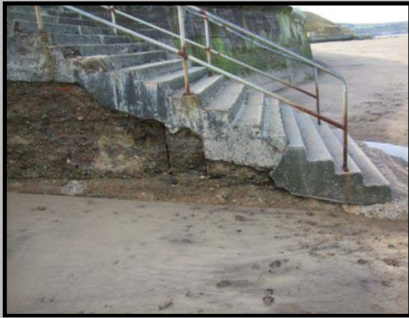
Erosion and cracking to stair side wall - image from 2009 (Asset Ref. 1221D901D0802C04001)
