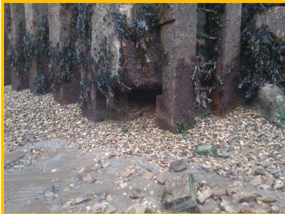
Void under SE corner of breakwater by lighthouse (Asset Ref. 1221D901D1301C17)
