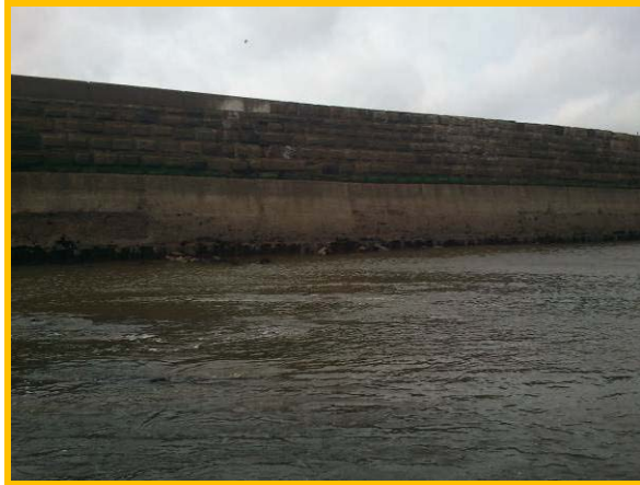
Area of displaced blocks on outer face of east pier (Asset Ref. 1221D901D0803C03)
