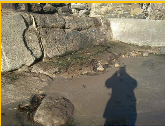
Wide cracks to toe of wall and undermining (Asset Ref. 1221D901D1003C06)
