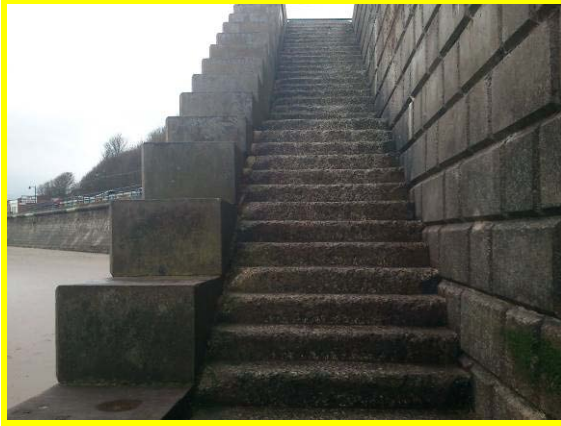
Exposed aggregate on access steps (Asset Ref. 1221D901D1602C04)
