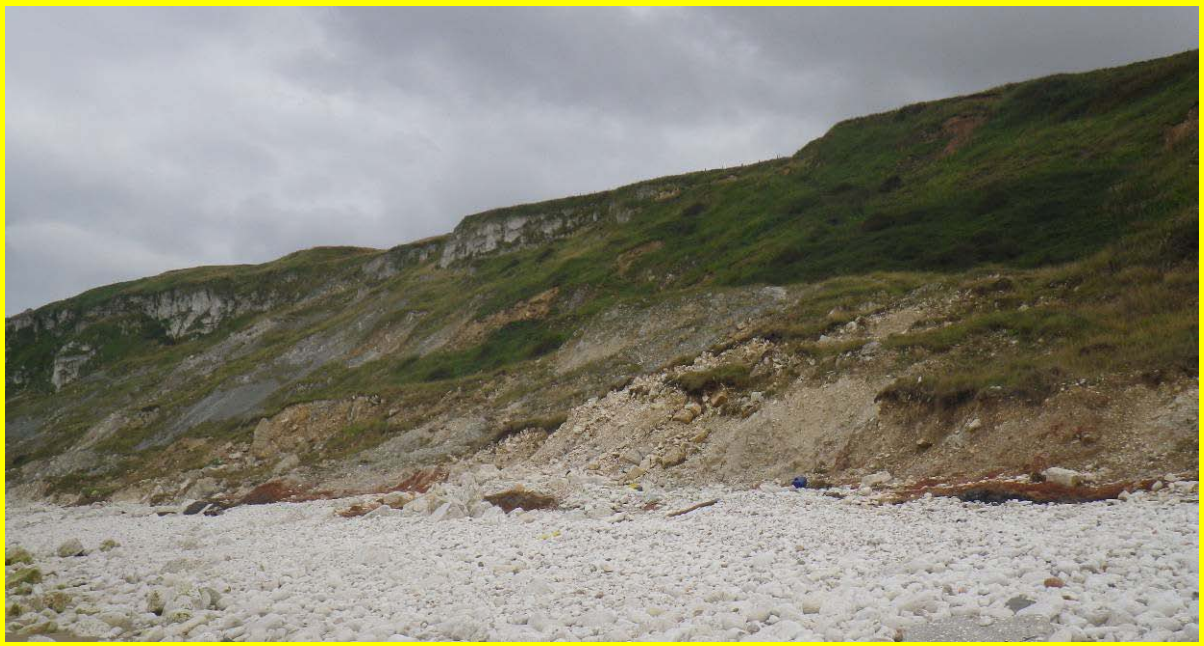
MU29/CJ Active toe erosion and localised mudsliding (Locally Active)
