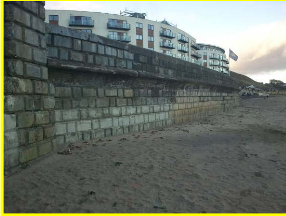
Abraded / eroded blocks and splash beam at Peasholm Gap. (Asset Ref. 1221D901D1201C19)
