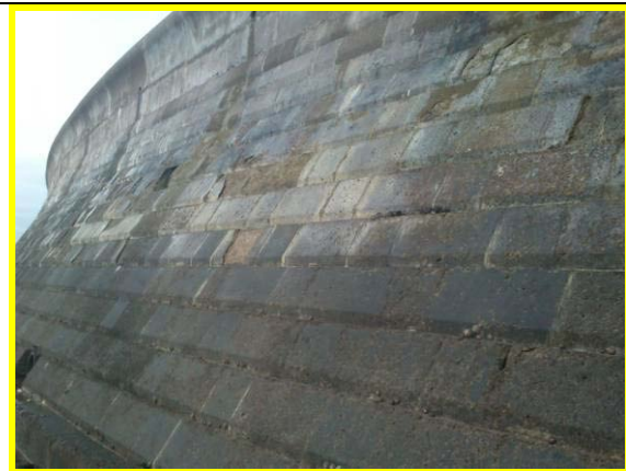
Damage to face of blocks on wall at Sea Life Centre (Asset Ref. 1221D901D1201C02)
