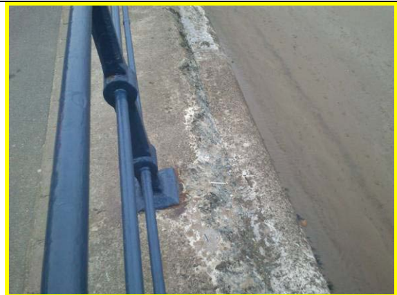
Damaged coping and splash beam (Asset Ref. 1221D901D1602C03)
