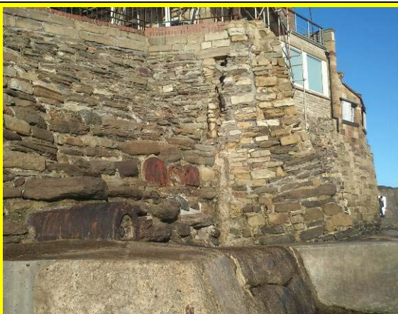
Cracks and missing stonework in upper wall (Asset Ref. 1221D901D1003C06)
