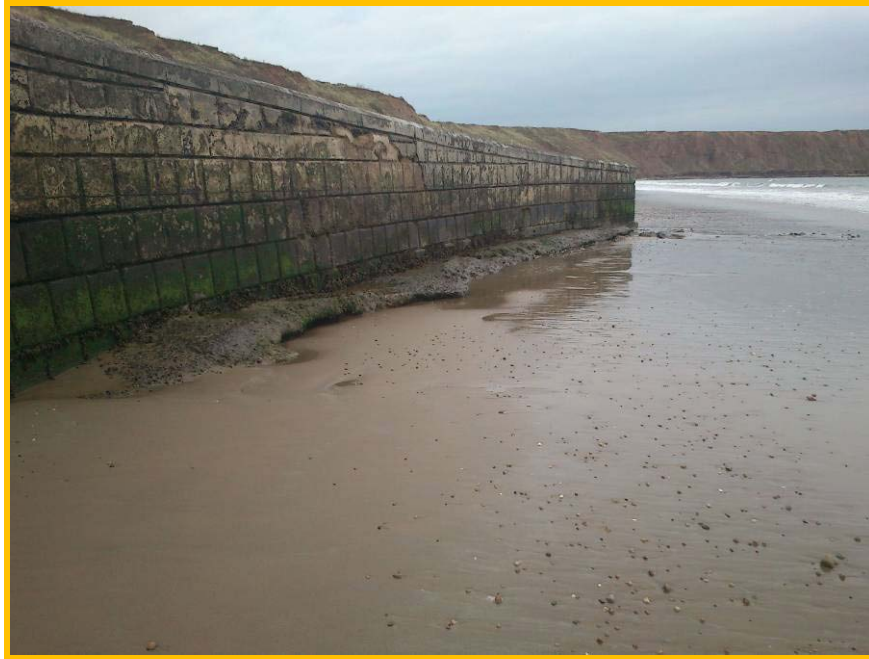
Exposed and undercut toe apron at Cobble Landing (Asset Ref. 1221D901D1602C09)
