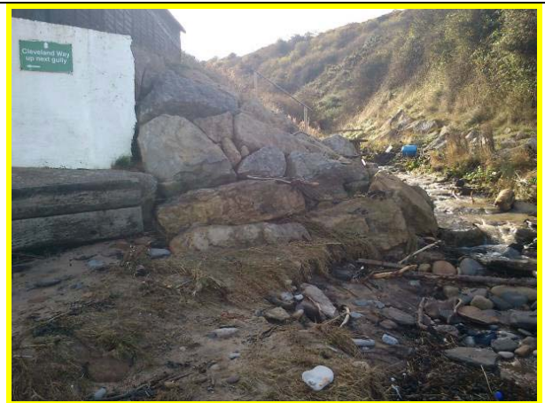
Northern end of defences at Runswick Bay sailing club (Asset Ref. 1221D901D0602C05)
