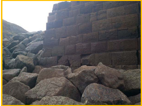
Loose blocks at south outer end of east breakwater (Asset Ref. 1221D901D0803C03)
