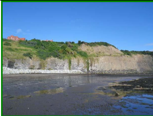
MU16/2 The cliffs have been stabilised at the toe but show some signs of erosion on their face (Dormant).
