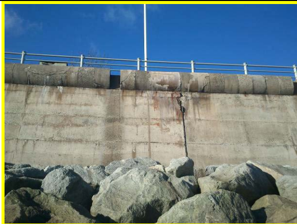
Quarter Deck sea wall with cracked capping beam with previous repairs (Asset Ref. 1221D901D1003C10)
