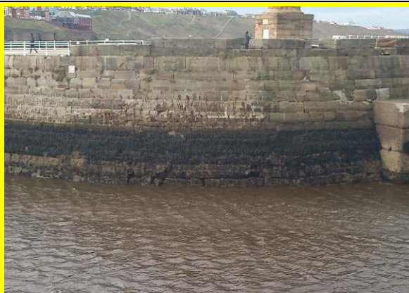
Missing blocks at LW line NE corner of West Breakwater (Asset Ref. 1221D901D0803C02)
