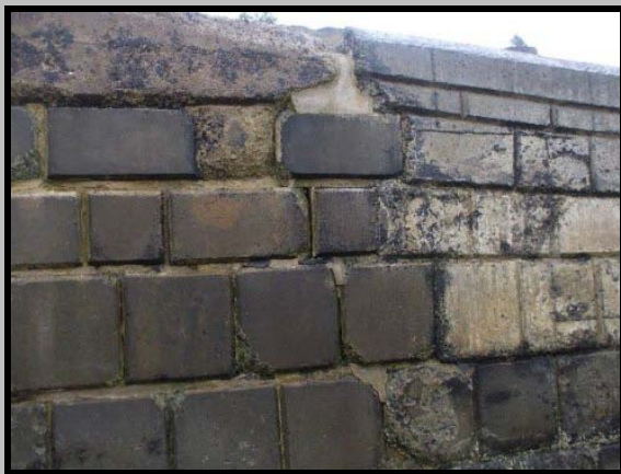
Photo from 2009 inspection of crack at Cobble Landing – (Asset Ref. 1221D901D1602C09)
