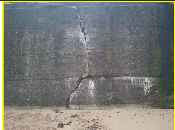
Vertical crack through wall (no change since 2009) (Asset Ref. 1221D901D0403C01)
