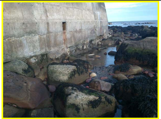
Foreshore scour at toe of seawall, photo from 30/10/2012 (Asset Ref. 1221D901D0601C01)
