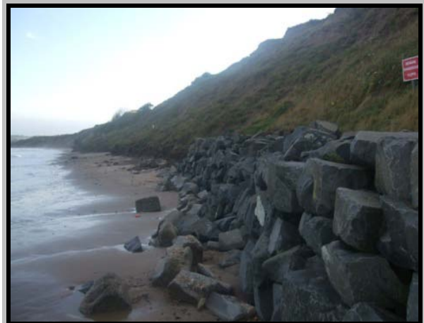
Rock revetment with gabion baskets beneath. Photo from 2009 inspections. (Asset Ref. 1221D901D1602C02)
