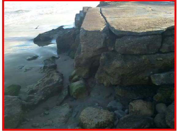
Voids beneath and failing front face at defence at beach access south of the pumping station (Asset Ref. 1221D901D1402C06)
