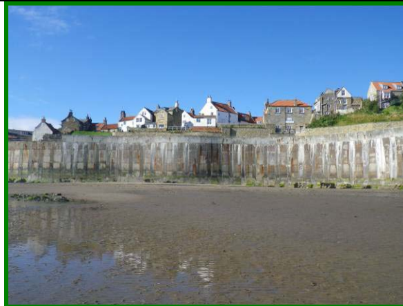
MU16/3 The cliff at this location has been stabilised and is not visible through much of the unit (Dormant).
