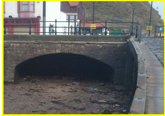
Spalling concrete capping to arched suspended quay at east end of Sandside (Asset Ref. 1221D901D1301C05)
