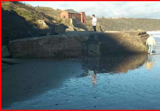
Difficult public access at failing beach defence (Asset Ref. 1221D901D1402C06)
