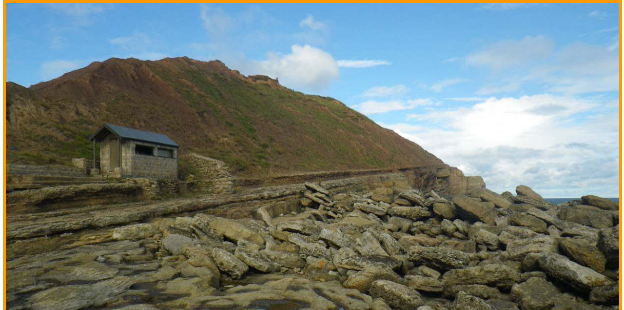
MU27/B The toe is protected to some extent but the cliff slope continues to erode (Partly Active)
