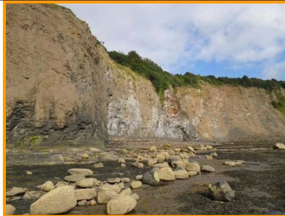
MU16/1 the base of the cliff continues to erode. The undercutting of the cliff is evident in the left side of the photograph (Partly Active)
