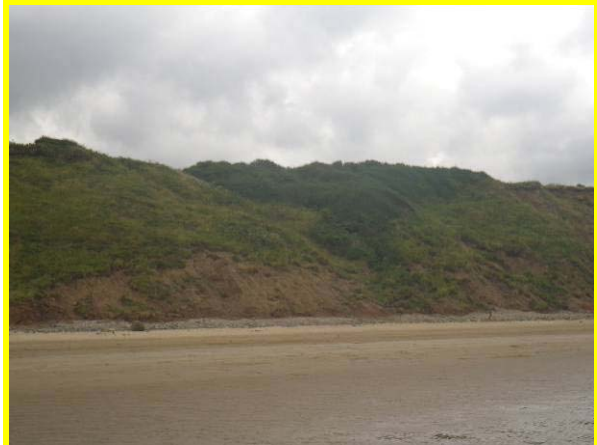
MU29/AH Heavily vegetated with toe erosion, which is severe in places (Locally Active)
