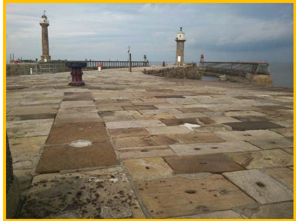
Open gaps between sandstone slabs in deck of east pier (Asset Ref. 1221D901D0803C03).
