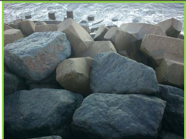
View of Accropode armour with concrete piles at toe and rock crest visible (Asset Ref. 1221D901D1202C02)
