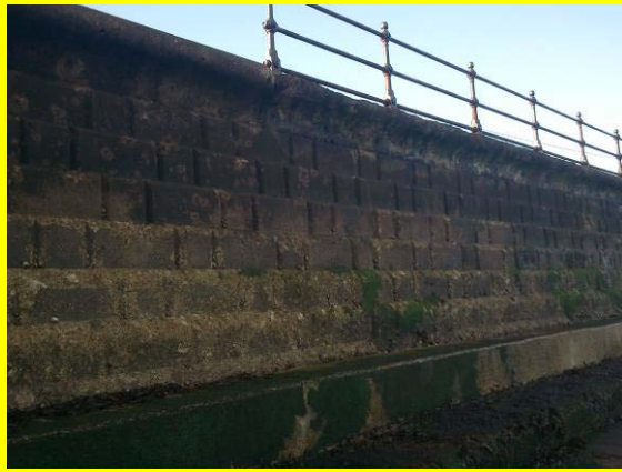
Erosion and spalling of front face of wall and exposed toe. Asset Ref. 1221D901D1201C03
