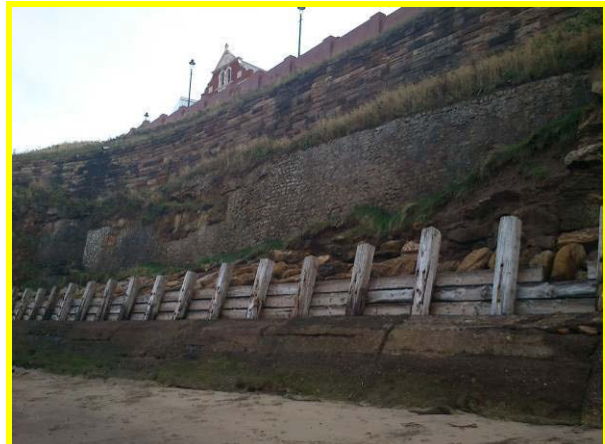
Mortar loss and surface erosion to middle and upper wall (Asset Ref. 1221D901D0802C05)
