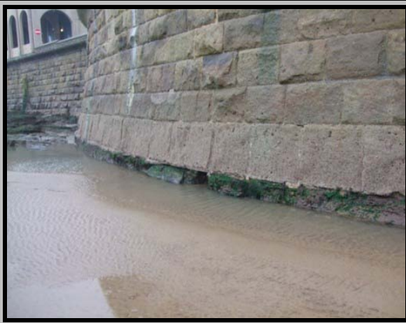
Undercutting to the sea wall – photo from 2009 (Asset Ref. 1221D901D1301C28)
