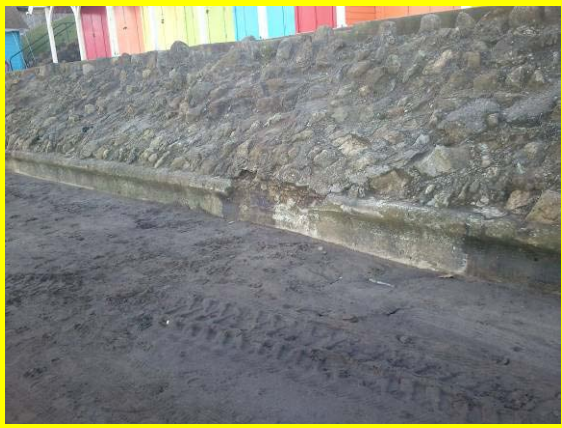
Damage to rear wall and grouted revetment (Asset Ref. 1221D901D1201C05)
