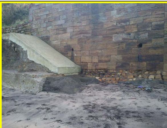
Visible joint washout and seepage (Asset Ref. 1221D901D0802C06)
