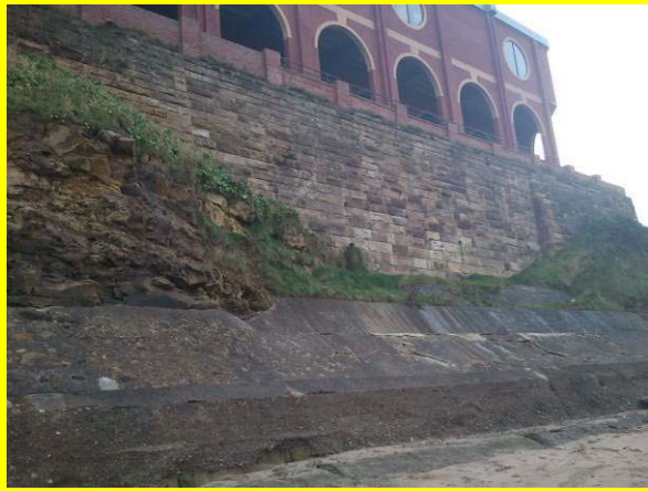
Cracking in concrete revetment toe. (Asset Ref. 1221D901D0802C15)
